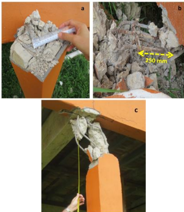
Fig. 4. Large spacing between stirrup in columns [19]
