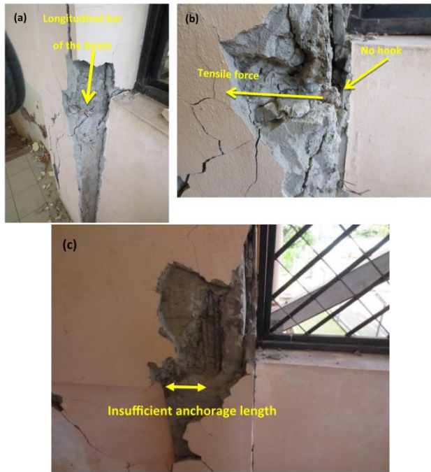
Fig. 6. The insufficiency of anchoring at the end of the reinforcing bar causes column damage [19].
